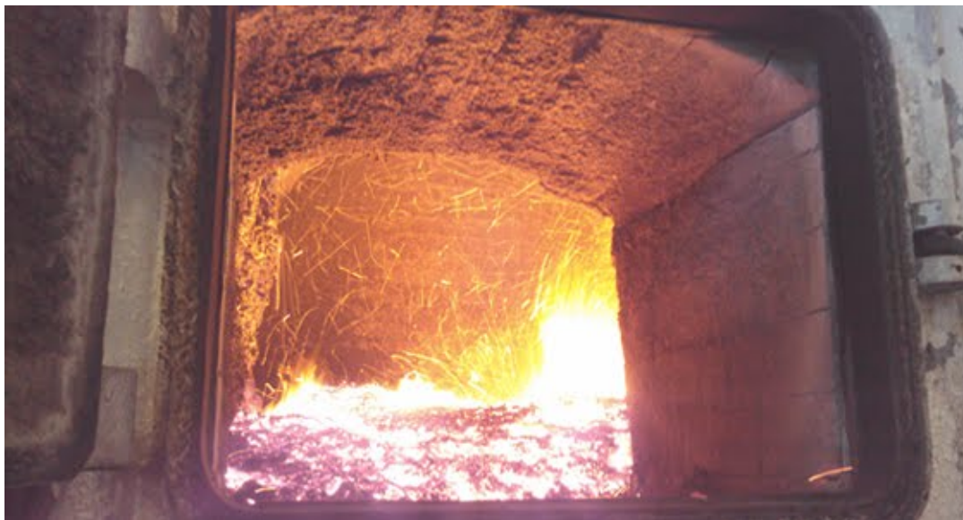
The boiler of the Piedmont Geriatric Hospital is now fueled with switchgrass, producing steam to heat the facility and saving the hospital $1300 a day compared to heating oil.
